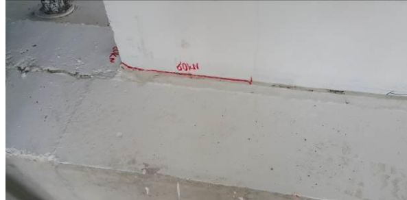
Figure 6. A thin crack line under a 60 kN.
