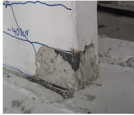
Figure 9. Bended sheet plate becoming visible in the shear wall end zones.
