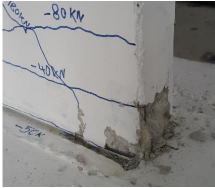
Figure 8. Crushing effects in the pressure zone.
