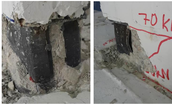
Figure 10. Buckling occurring in the bended sheet plates at the right end of the shear wall under 202 kN.
